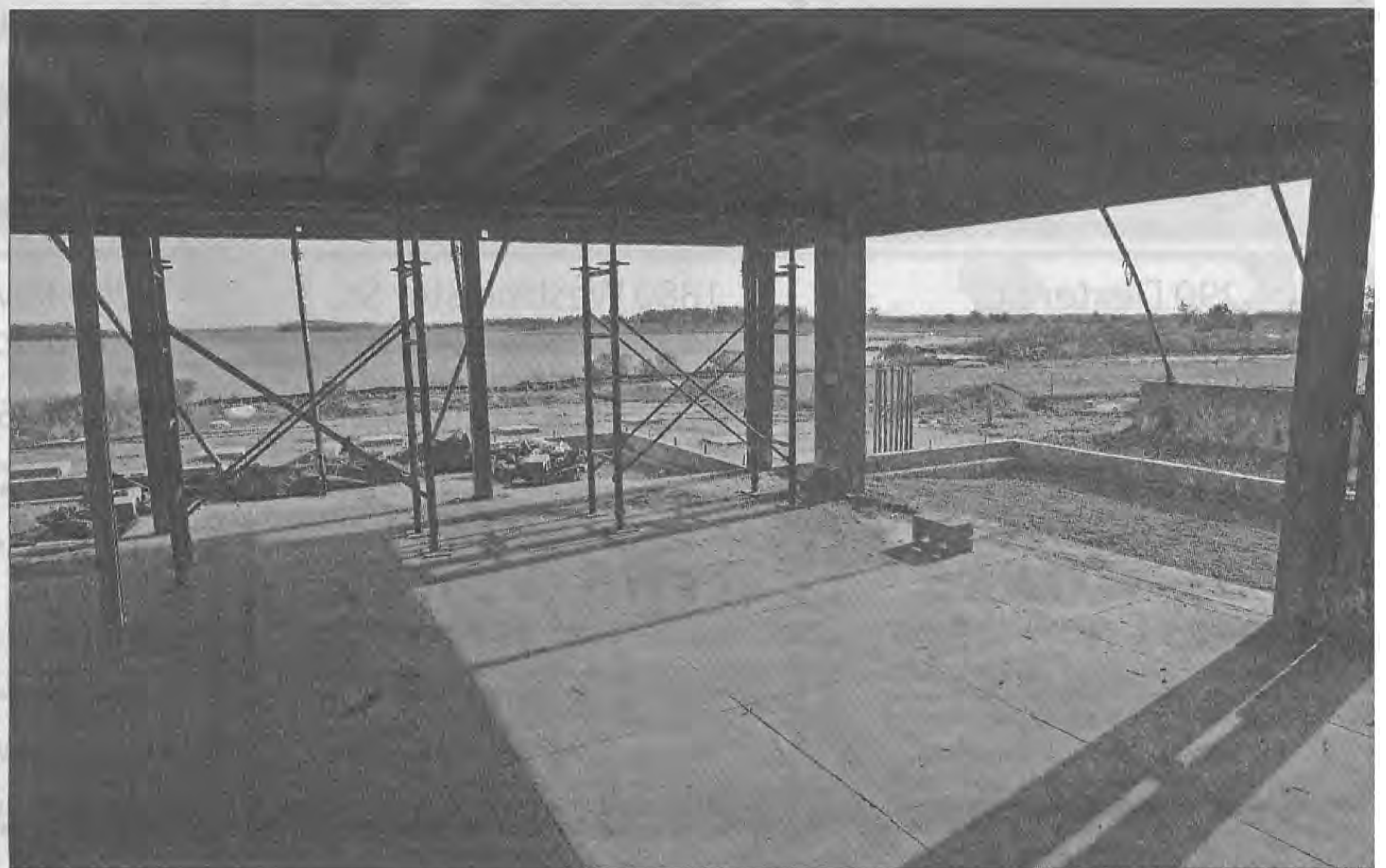
The space that will contain the new dining room of the Weekapaug Inn offers a view of the water and the countryside. The inn is being renovated by new owners Langdon Wheeler and Charles Royce. They are planning on opening in October of next year.
