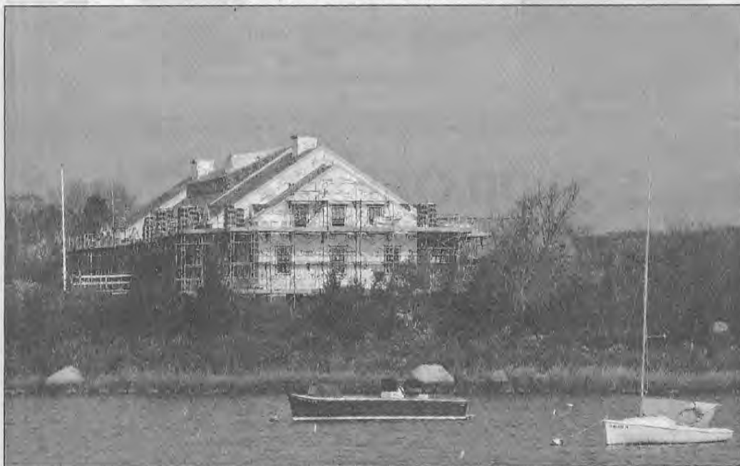
A view of the inn with renovation construction framing visible as seen from across Weekapaug Pond.
